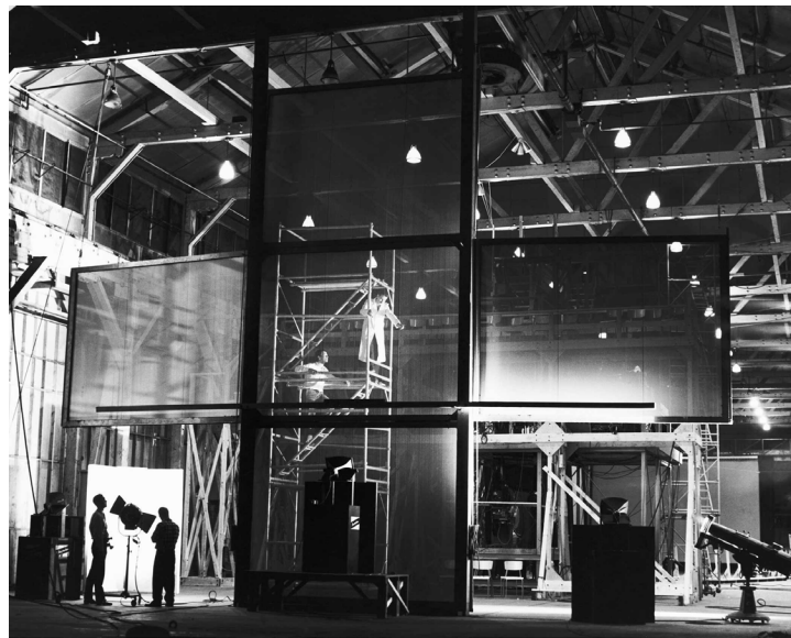
Photograph of the construction of the multi-screen in the third room of the Labyrinth pavilion. See database entry.
